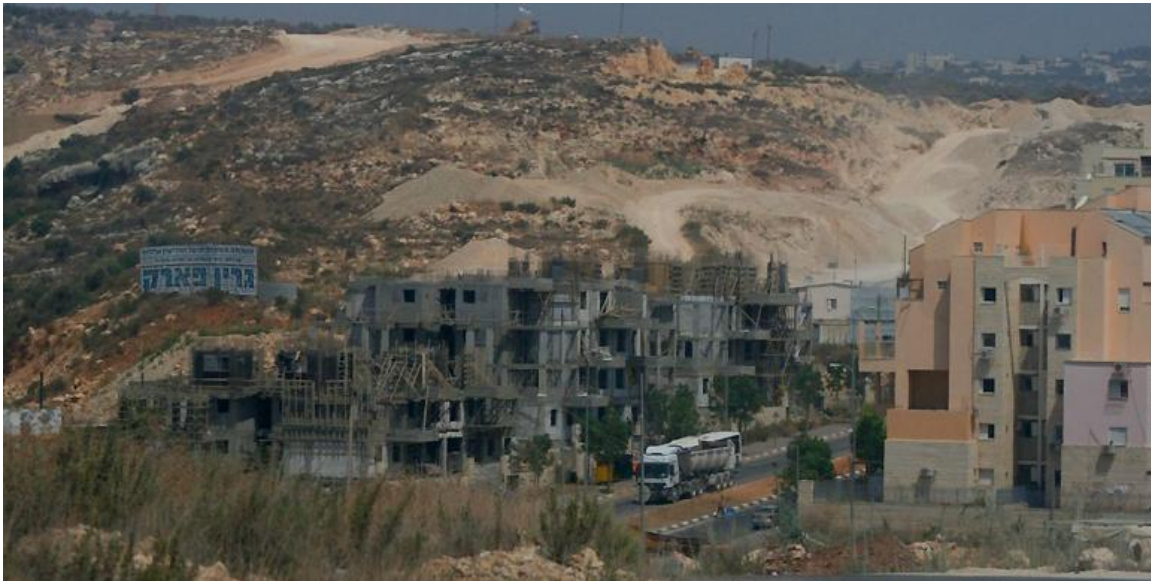
Modi'in Ilit (near Ramallah) – The Canadian company Green Park advertising its properties under construction. August 2010 – Al-Haq©
