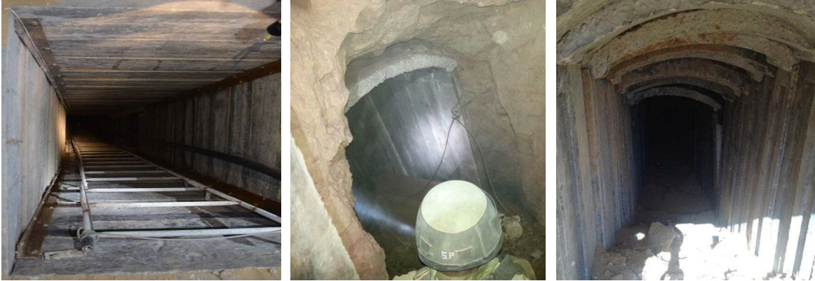
Above: Photos of tunnels found during the ground operation phase of the 2014 Gaza Conflict (Source: IDF). 46
