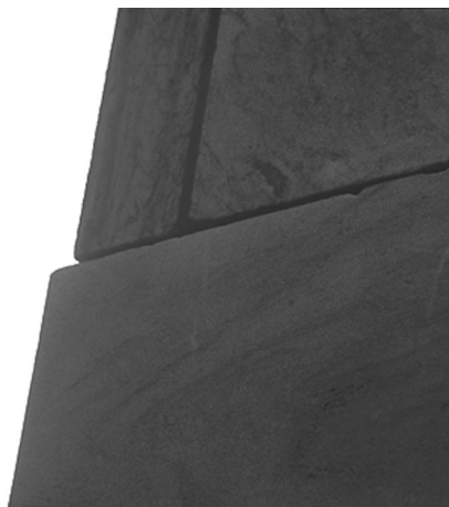
Figure 6: Stone Displacement Due to Effects of Age
